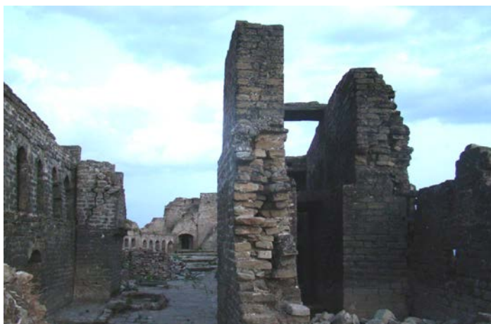
Fig. 9 Main Face of The Dilapidated Wall, Giving First Glimpse of The Fort
