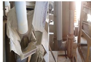
Fig. 2 Dust suction point and blower
