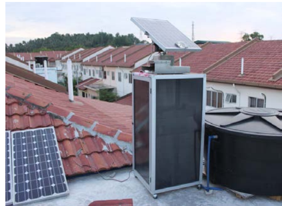
Fig. 1: Data Logger Location and Set-up
